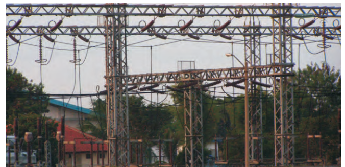
Project Name : TRANSMISSION TOWER 500 KV Client Name : PT. PLN (Persero) Pikitring JBN Tonnage : 2.750 MT Location | Year : Tasikmalaya, West Java - Indonesia | 2007
