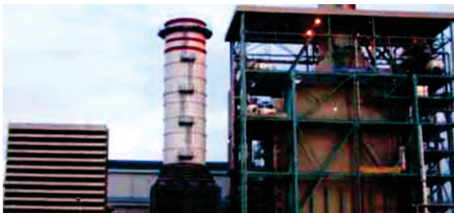
Project Name : PLTGU PALEMBANG 150 MW Client Name : PT. Asrigita Prasarana Tonnage : 409 MT Location | Year
