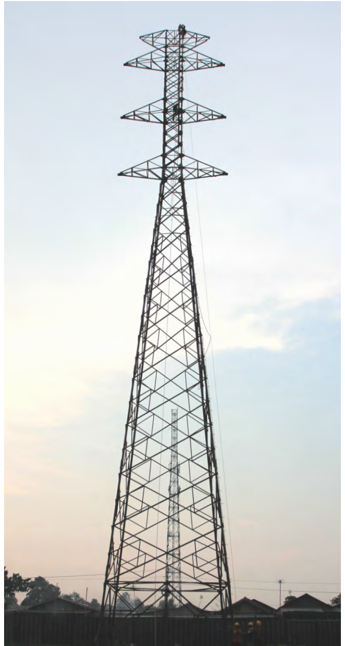
Project Name : TRANSMISSION TOWER 150 & 500 KV Client Name : PT. PLN (Persero) Pikitring JBN Tonnage : 14.000 MT Location | Year : Semarang, Central Java - Indonesia | 2003
