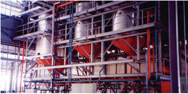
Project Name : CRUDE PALM OIL (CPO) MILL Client Name : PT. Bumi Sarima Kelapa Tonnage : 50 MT Location | Year : Padang, West Sumatera - Indonesia | 2000
