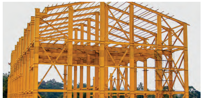
Project Name : PLASTIC FACTORY Client Name : PT. Anta Tirta Kharisma Tonnage : 800 MT Location | Year : Sukabumi, West Java - Indonesia | 2017
