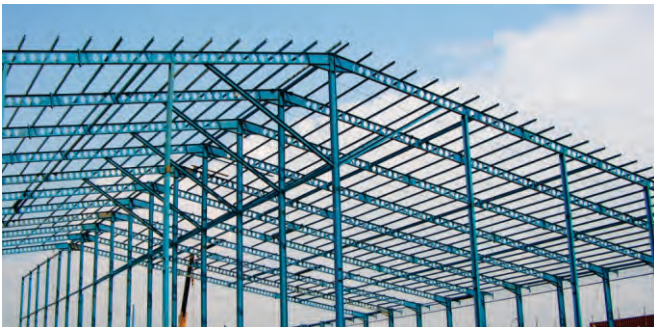
Project Name : SANEX FACTORY Client Name : PT. Sanex Qianjiang Motor Int. Tonnage : 1.300 MT Location | Year : Bekasi, West Java - Indonesia | 2000
