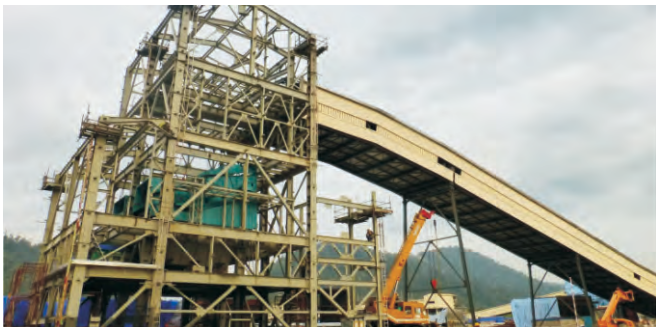
Project Name : TRANSFER TOWER Client Name : PT. Semen Cibinong Tonnage : 104 MT Location | Year : Cibinong, Bogor, West Java - Indonesia | 2006
