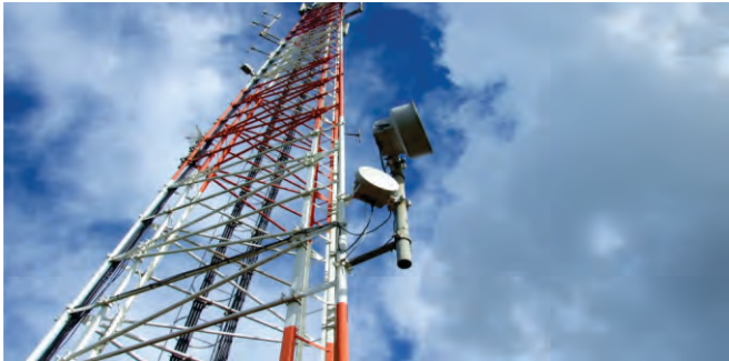
Project Name : TELECOMMUNICATION TOWER Client Name : PT. Bahayutama Kerta Mukti Tonnage : 46 MT Location | Year : Jakarta - Indonesia | 2003
