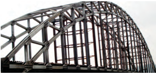
Project Name : JEMBATAN PELENGKUNG A-128 Client Name : PT. Fajar Parahyangan Tonnage : 600 MT Location | Year : Bojonegoro, Central Java - Indonesia | 2006
